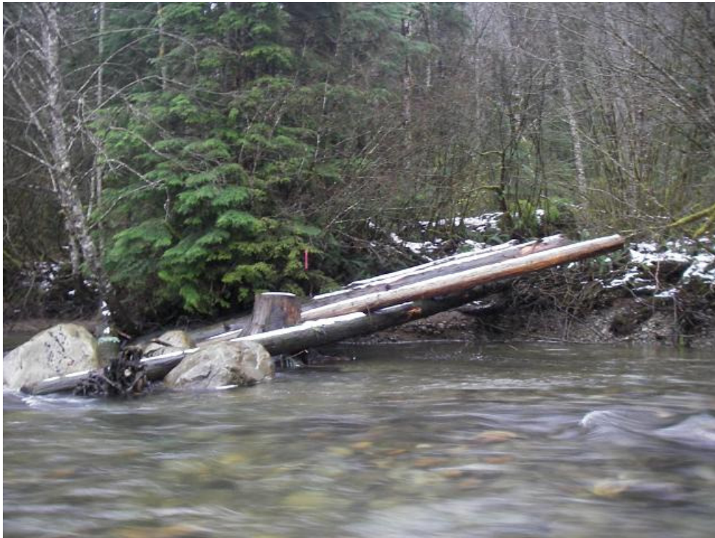
Figure 1: LWD structure upstream of Spur 6 access point; high river levels eroded a portion of the bank behind the downstream primary log.
